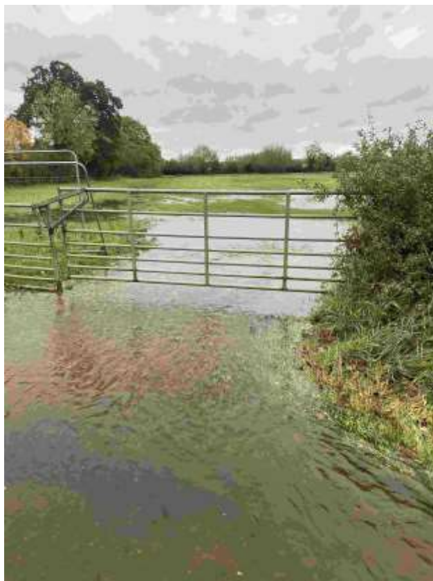
Water flooding east into the field between the culvert and the railway bridge
